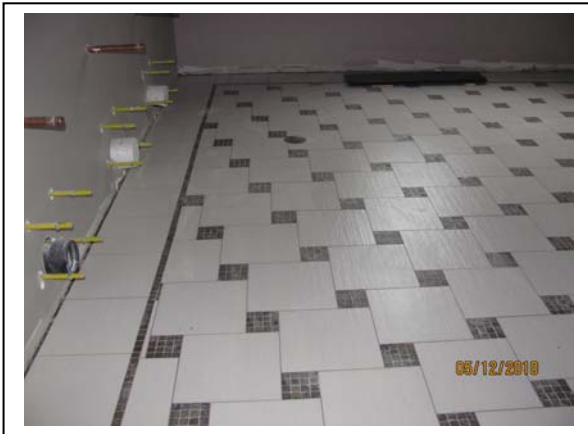
Incorrect layout - to be removed
